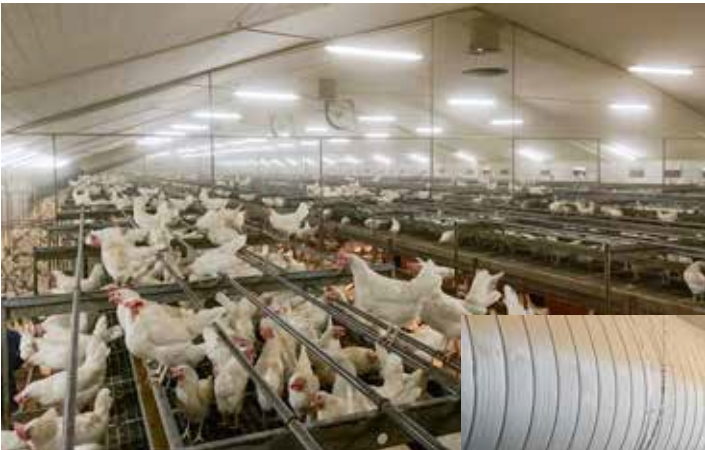
The air from the heat exchanger is blown into the middle of the house and distributed through a series of ventilators
