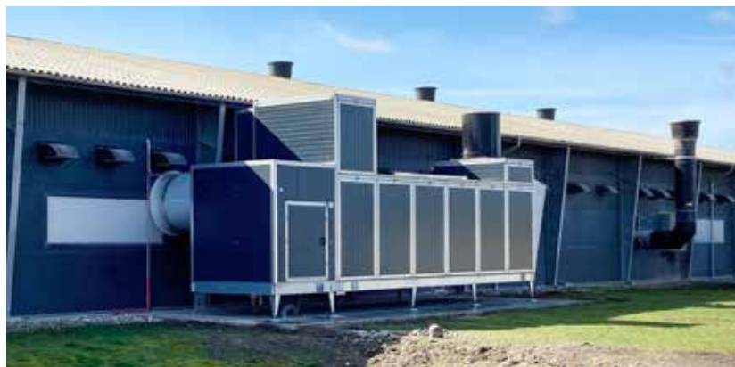
The heat exchanger from Agro Supply outside the hen house at Jens Skovgaard's farm
